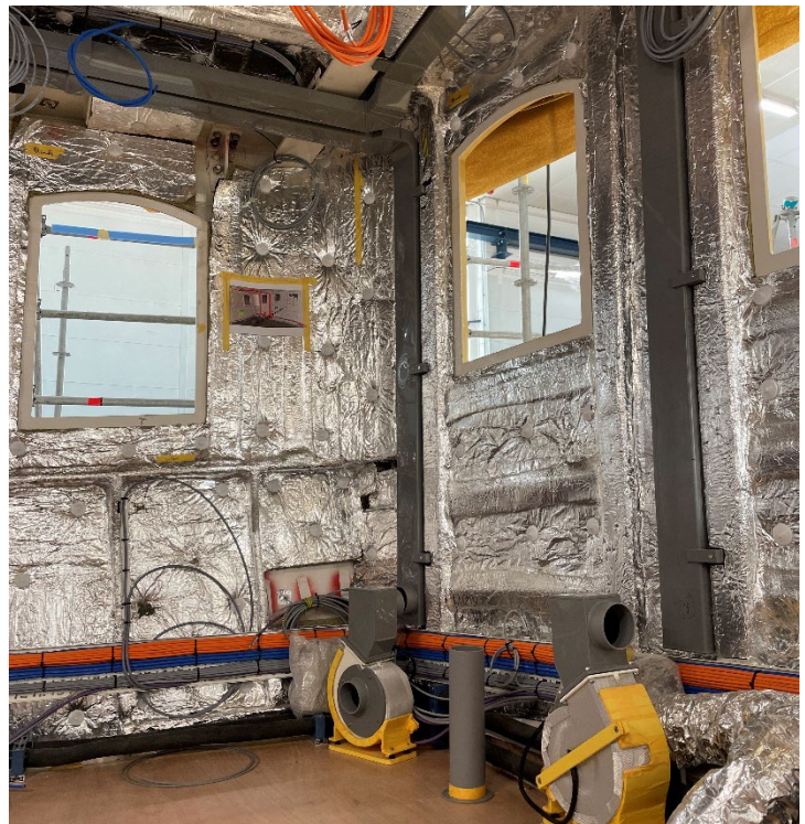
SQUARE HVAC DUCTING IN THE SALON AND MEDIA LOUNGE
